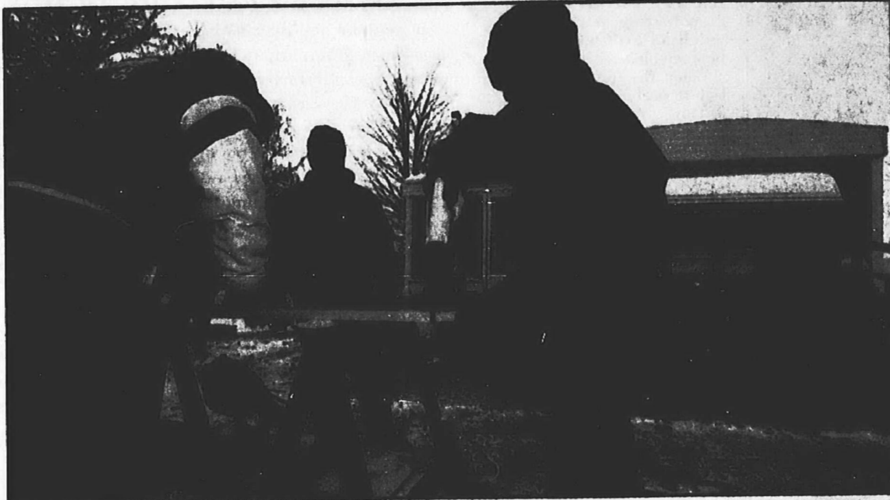
Helping hands: Plymouth Rotarian Paul Dillon, right, cuts a board as John Folino, left, lends a hand. The Rotarians, along with some help from Horton Plumbing, assembled a handicap ramp in front of the trailer of Steve and Terry Buentello. Kirk Kohn is at rear, watching.
