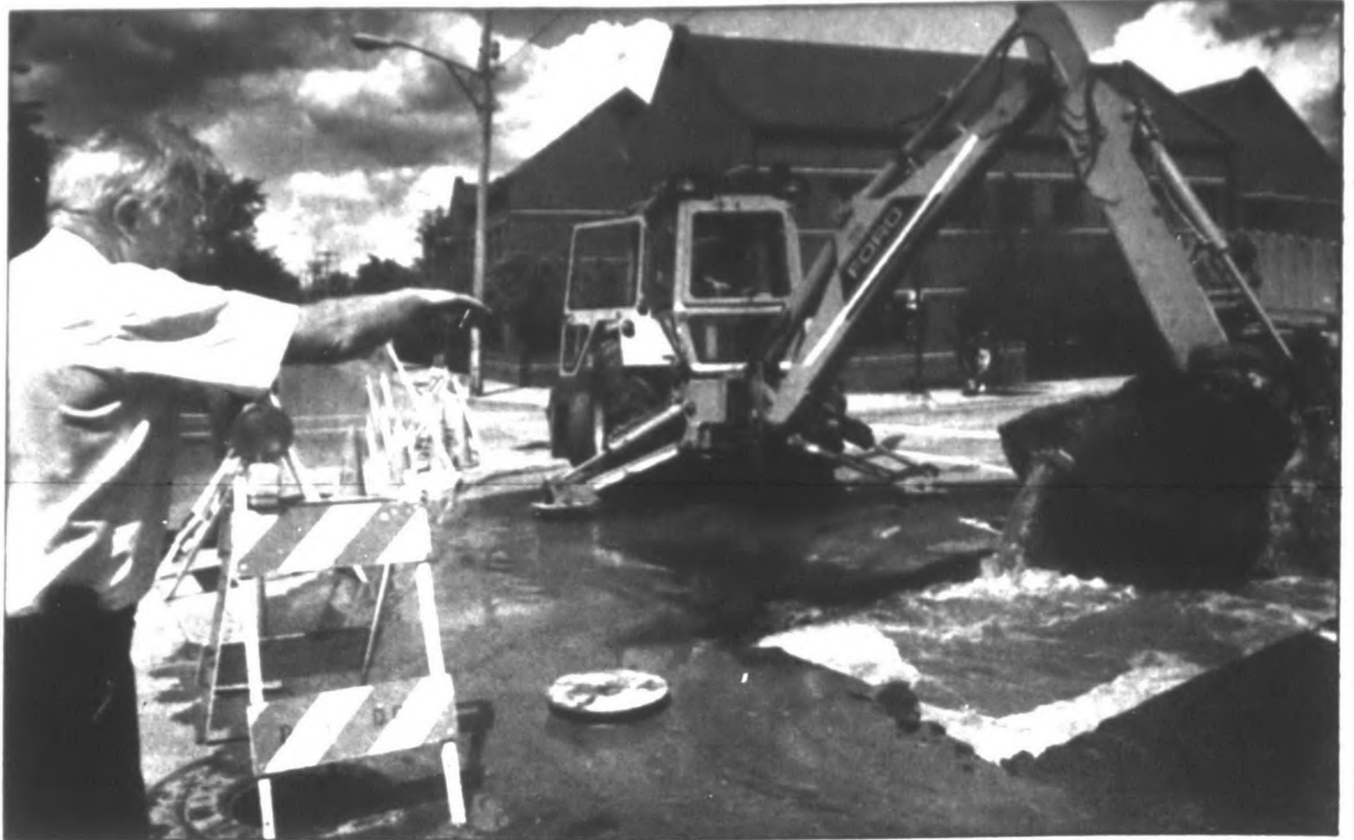
Street floods: Mel Behling of the department of public works gestures toward the intersection of Ann Arbor Trail and Harvey where the rupture of an aging 6-inch water main at about 3 p.m. Tuesday forced street closings. Water customers in about a two-block radius lost water, but DPW Director Paul Sincock said water was restored by 7 p.m. DPW crews rebuilt the manhole Wednesday. To allow cement to harden, the road will remain closed through today or Friday, Sincock said. A new cement patch is planned for the street in about two weeks.
