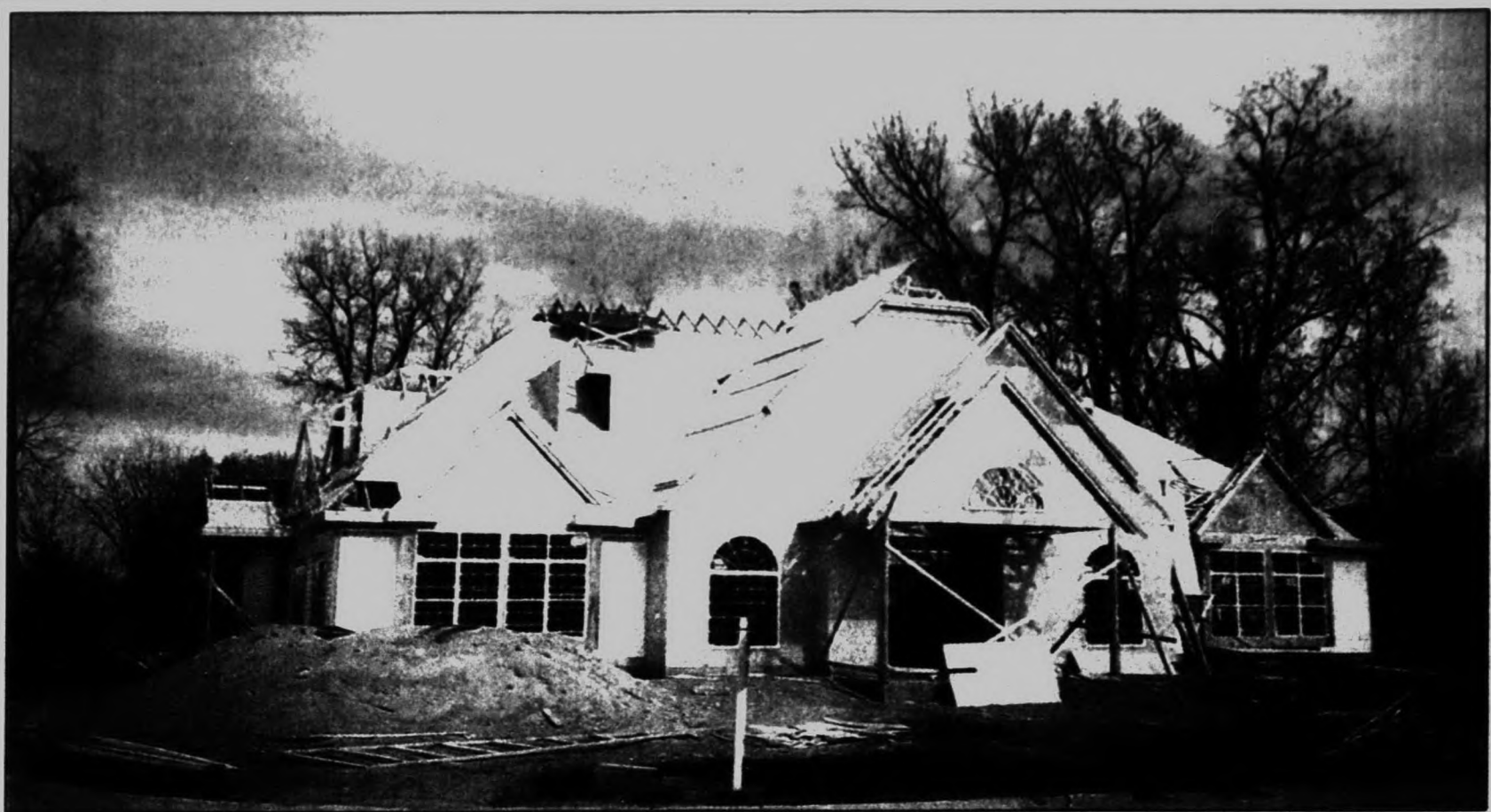
New amenity: Clubhouses, like this one under construction at Village Park of Beverly Hills, can add a new luster to older apartment complexes.
