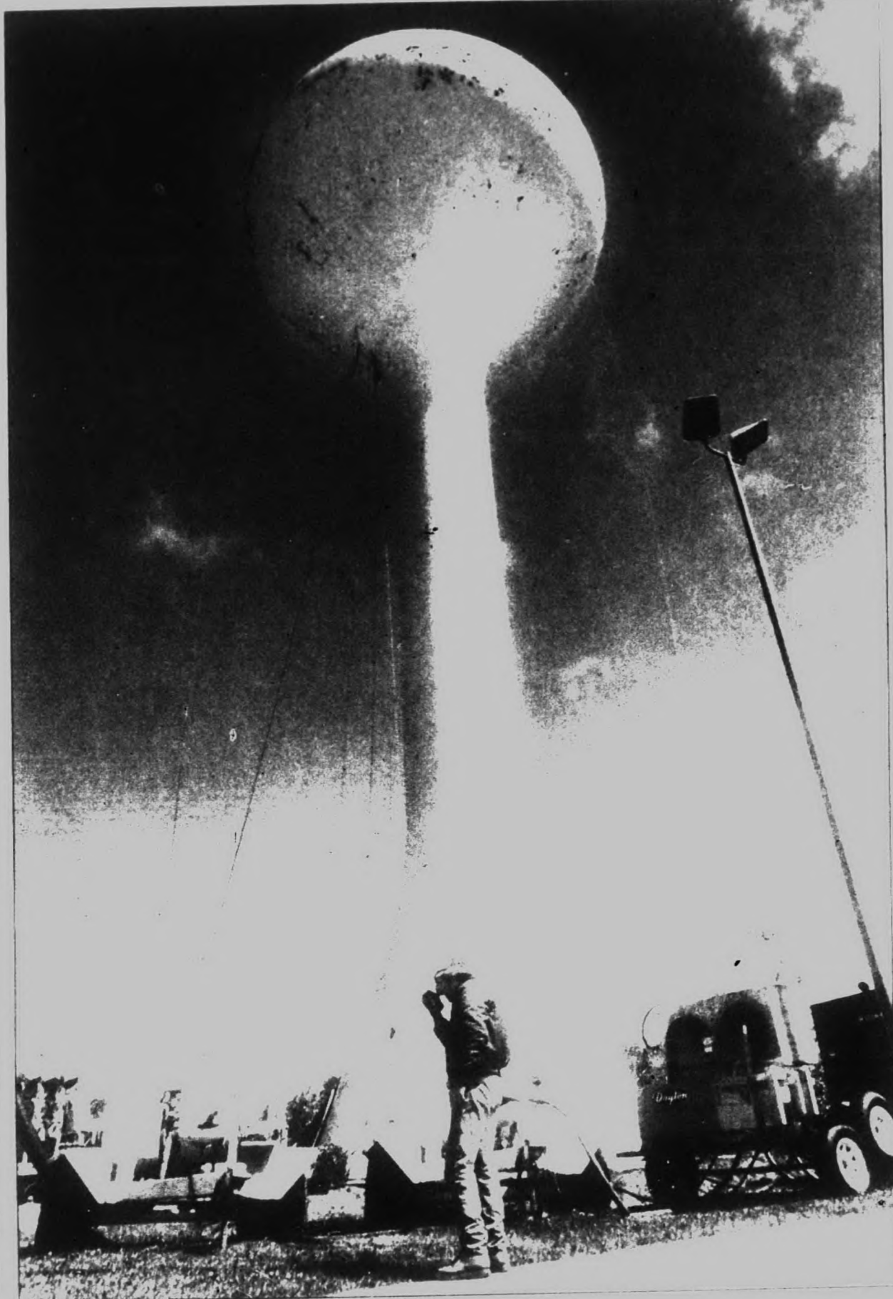
Sandblasting: One of the workers used a crew from Dixon Engineering to sandblast the Plymouth auto tower near M-14 to remove rust and prepare the structure for painting. Dixon used a portable, high-pressure sandblasting machine to blast the tower.
