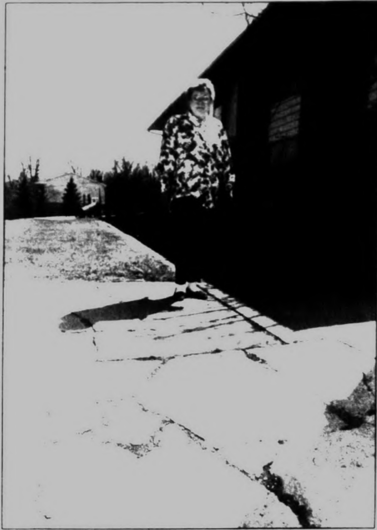
Work needed: Rita Lanci, who lives at the Mayflower, says city commission on Monday that repairs are needed throughout the complex.
