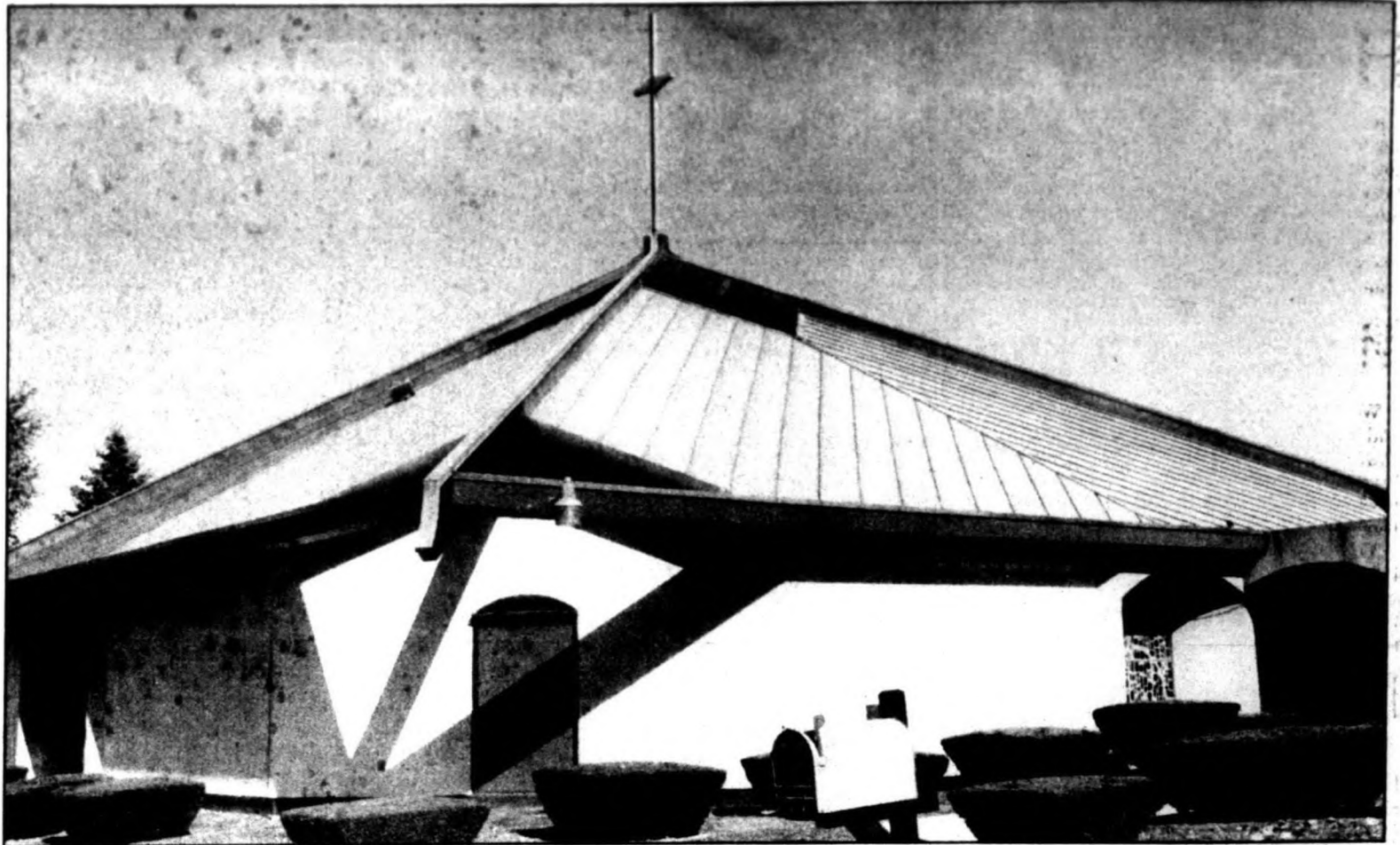
Durable design: Clarenceville United Methodist Church in Livonia is a gentle church reflecting the personality of former minister Elsie Johns, who worked with Brown Associates on its design back in the 1960s.
