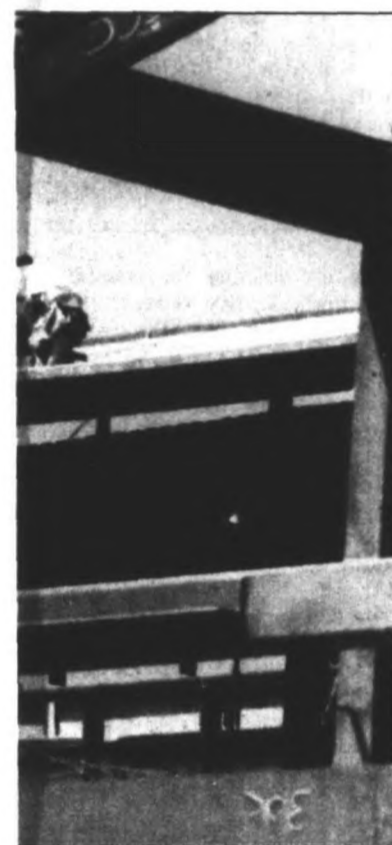
GUY WARREN/STAFF PHOTOGRAPHER View of the structure of the building in November.
