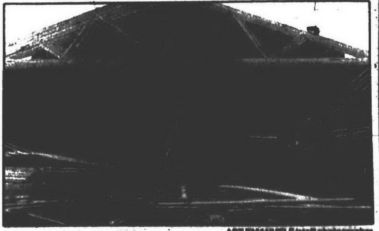
Five construction workers were injured when several roof trusses and two walls collapsed on this building under construction on Block Street in Garden City.
