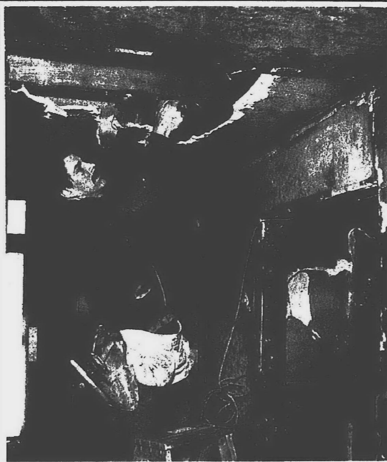
John Zap of J&J Electric checks the wiring in a hallway outside the Honeytree apartment which was destroyed by fire on Monday.
