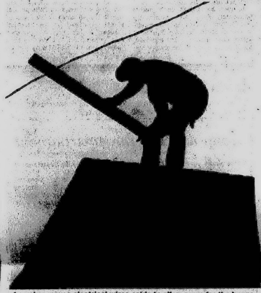
A worker moves electrical wires aside to allow room for the house to move underneath.
