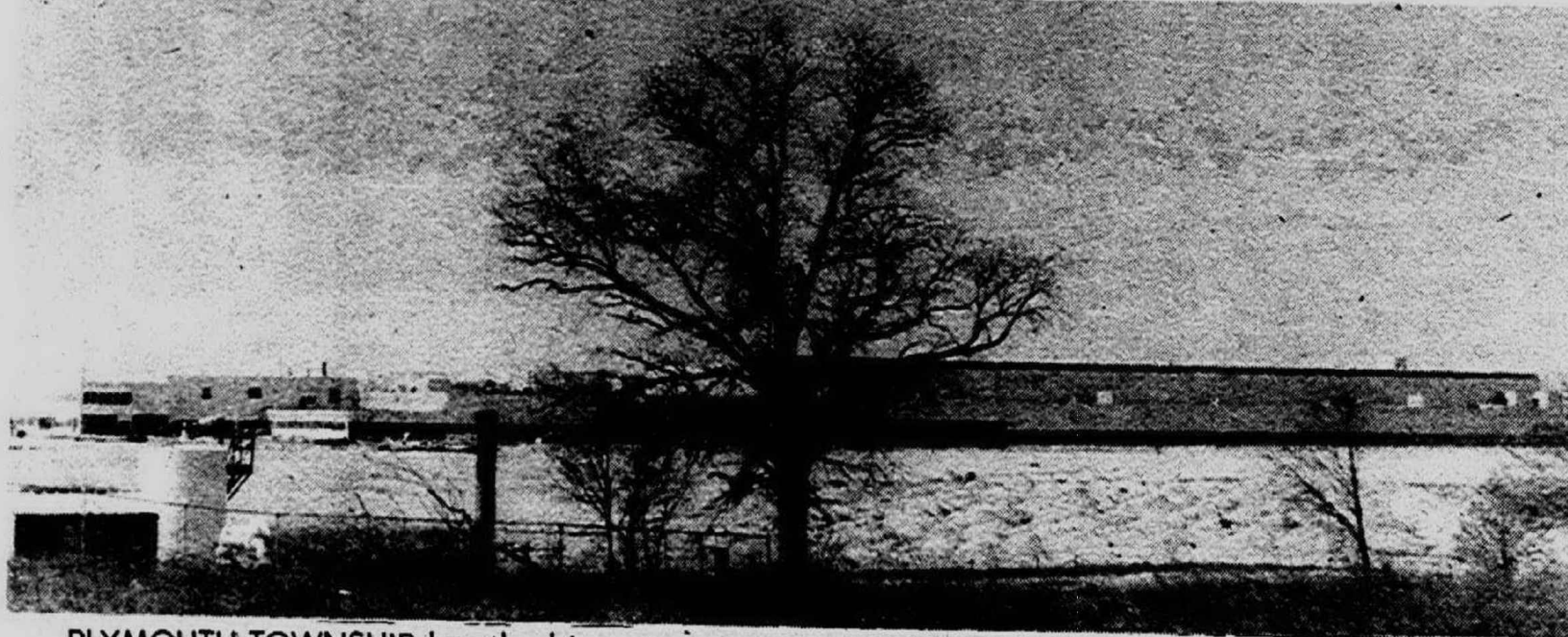
PLYMOUTH TOWNSHIP has the biggest construction project going in westurbia — a $5.5 million Ford Motor Co. plant on Sheldon Road
