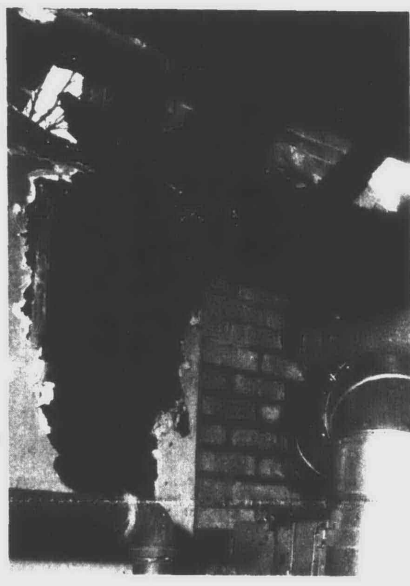
HERE'S EVIDENCE OF DAMAGE: The fire that swept through the Pilgrim Apartments last Saturday did considerable damage despite the great work of the firemen. One of the walls is shown here with a monster hole close to the chimney.
