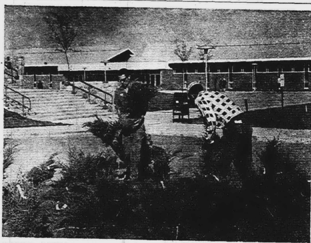
CAMPUS LANDSCAPING BEGINS — Workmen set one group of the nearly 200 low spreading junipers to be planted as part of a major landscaping program underway at the 139 acre Schoolcraft College campus. This first phase of the beautifica-
