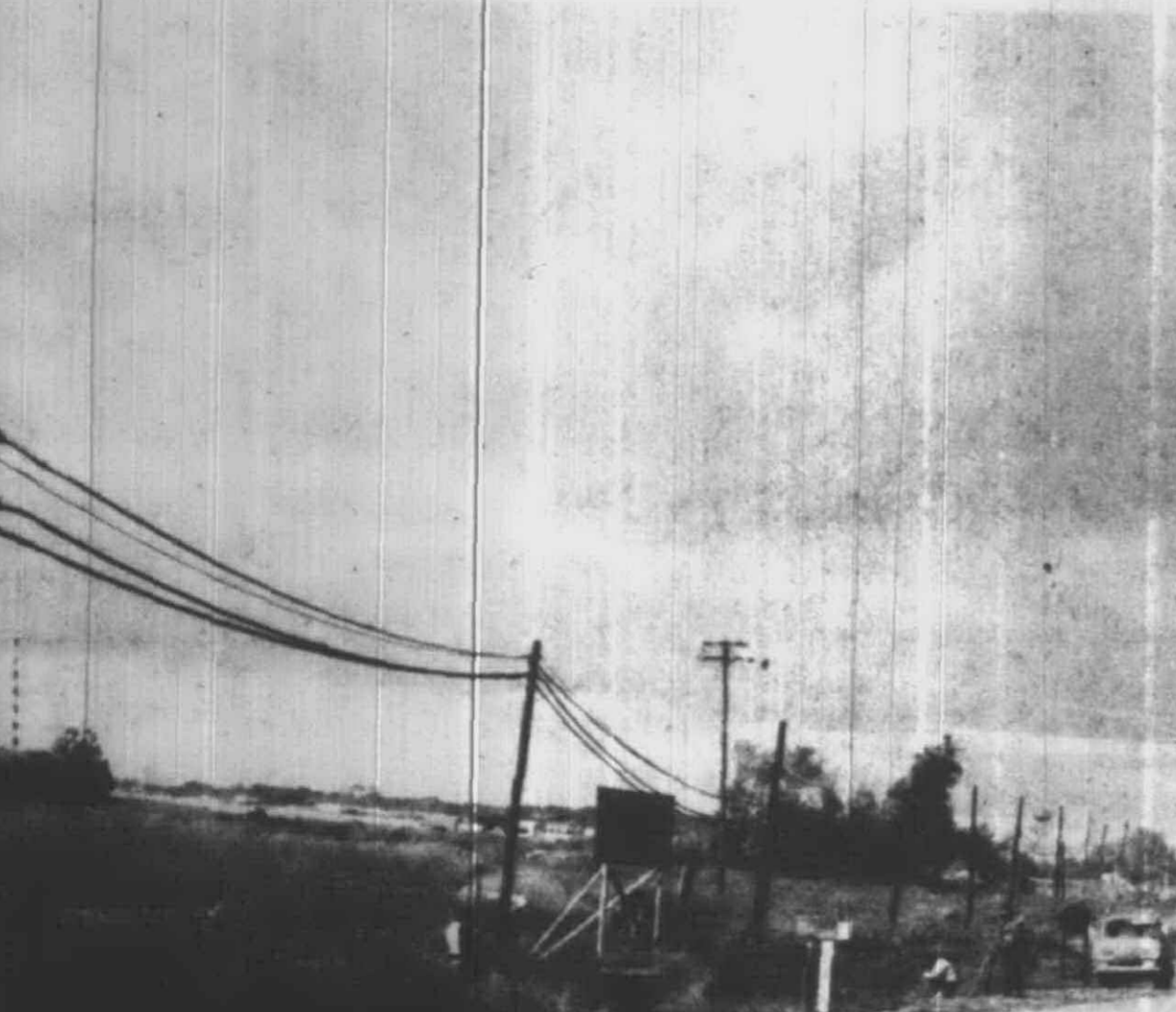
SHELDON ROAD widening project is underway as survey crews stake out the new right of way. Last week, utility poles were being moved in preparation for the soon-to-come closing of Sheldon from the C&O tracks to Five Mile Rd.
