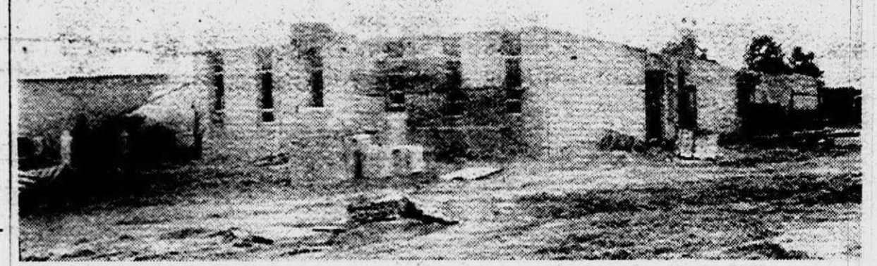
WILL IT BE FINISHED? This picture shows the progress on construction of elementary school No. 7 in the Plymouth School District which is scheduled for opening in September. There isn't any question that the early summer strikes delayed work but school officials have no idea at this time when the building will be ready for classes. They are hoping for October but have their fingers crossed.
