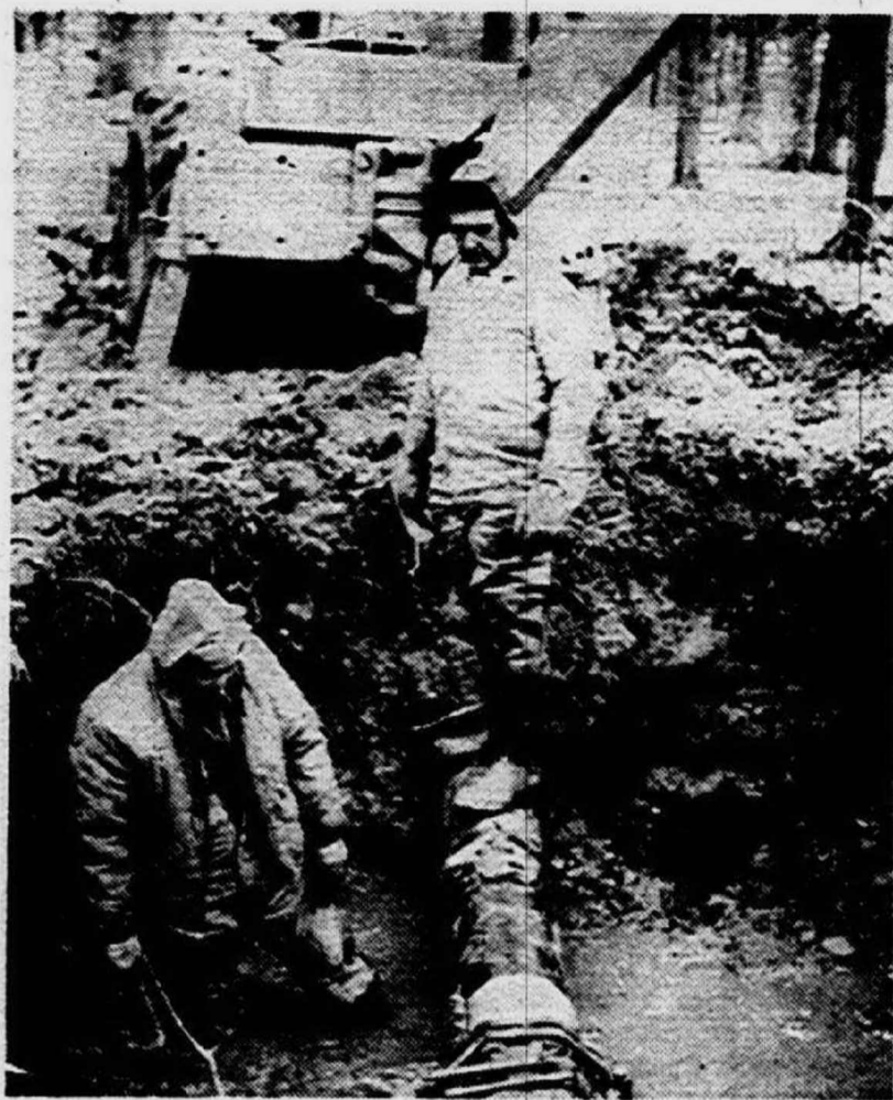
TROUBLE ON TROUBLE. That's what workers for the Plymouth Department of Public Works are thinking these days. A crew is shown in knee deep mud and water repairing the most recent 10-inch water main break near the comfort station in Cass Benton Park. The huge hole shows how much work was involved in stopping the leak.
