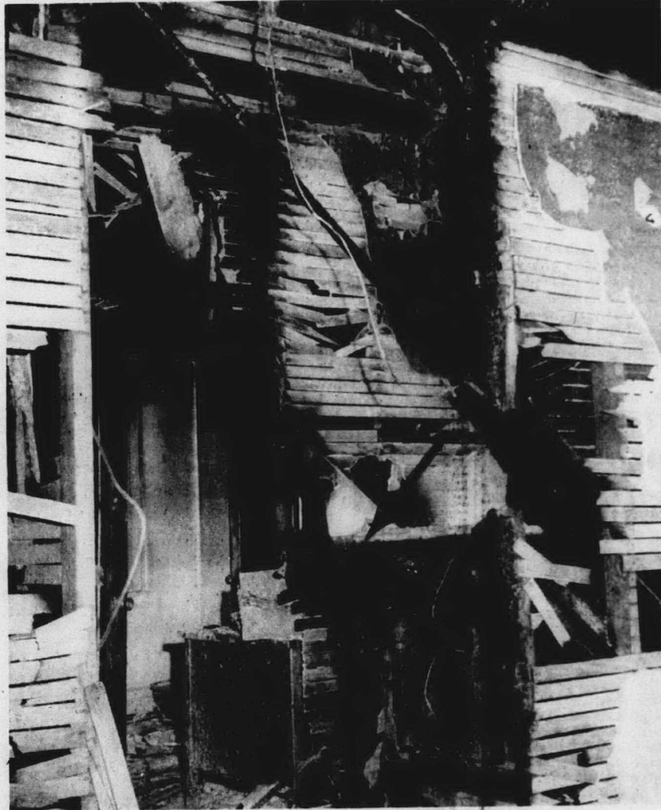
ONLY CHARRED timbers of what was once a stairwell (arrow) remain after fire gutted the interior of this home at 46985 N. Territorial Rd. late Monday afternoon. A neighbor summoned Plymouth Township firemen, who report the family of Eugene Johanningsmeir was vacationing in Indiana at the time. (See other pictures, Page A-8.)
