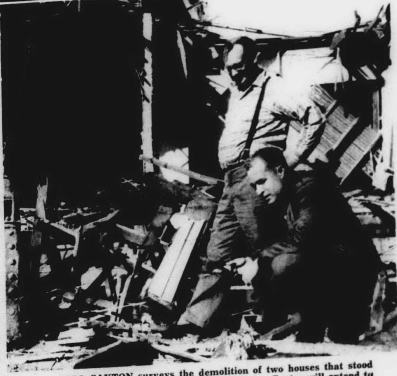
BILL SAXTON surveys the demolition of two houses that stood on the site of his new addition. Saxton's Garden Center will extend to Maple Street, and will have an alleyway along side, running from Ann Arbor Trail to Maple St.
