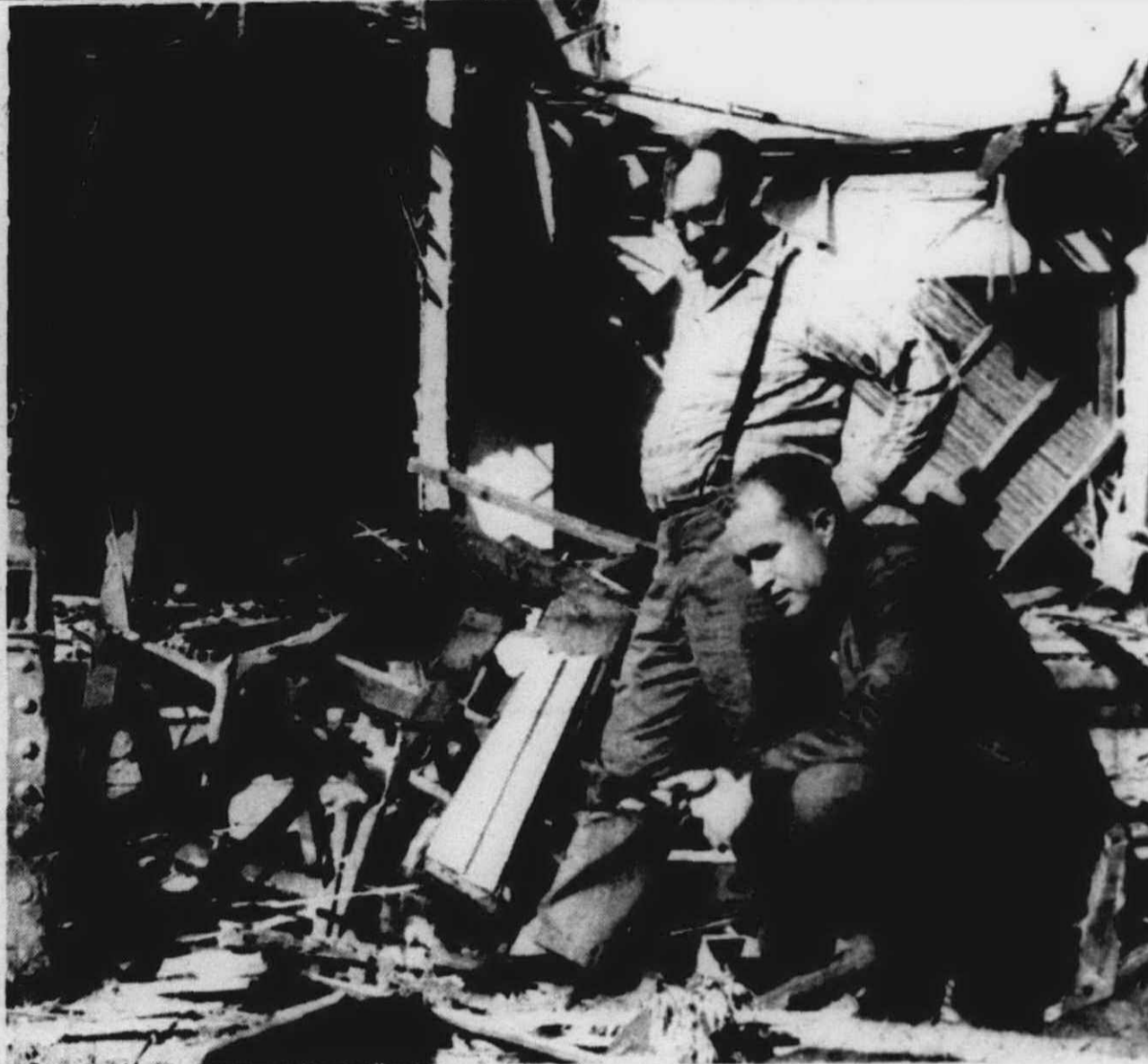
BILL SAXTON surveys the demolition of two houses that stood on the site of his new addition. Saxton's Garden Center will extend to Maple Street, and will have an alleyway along side, running from Ann Arbor Trail to Maple St.
