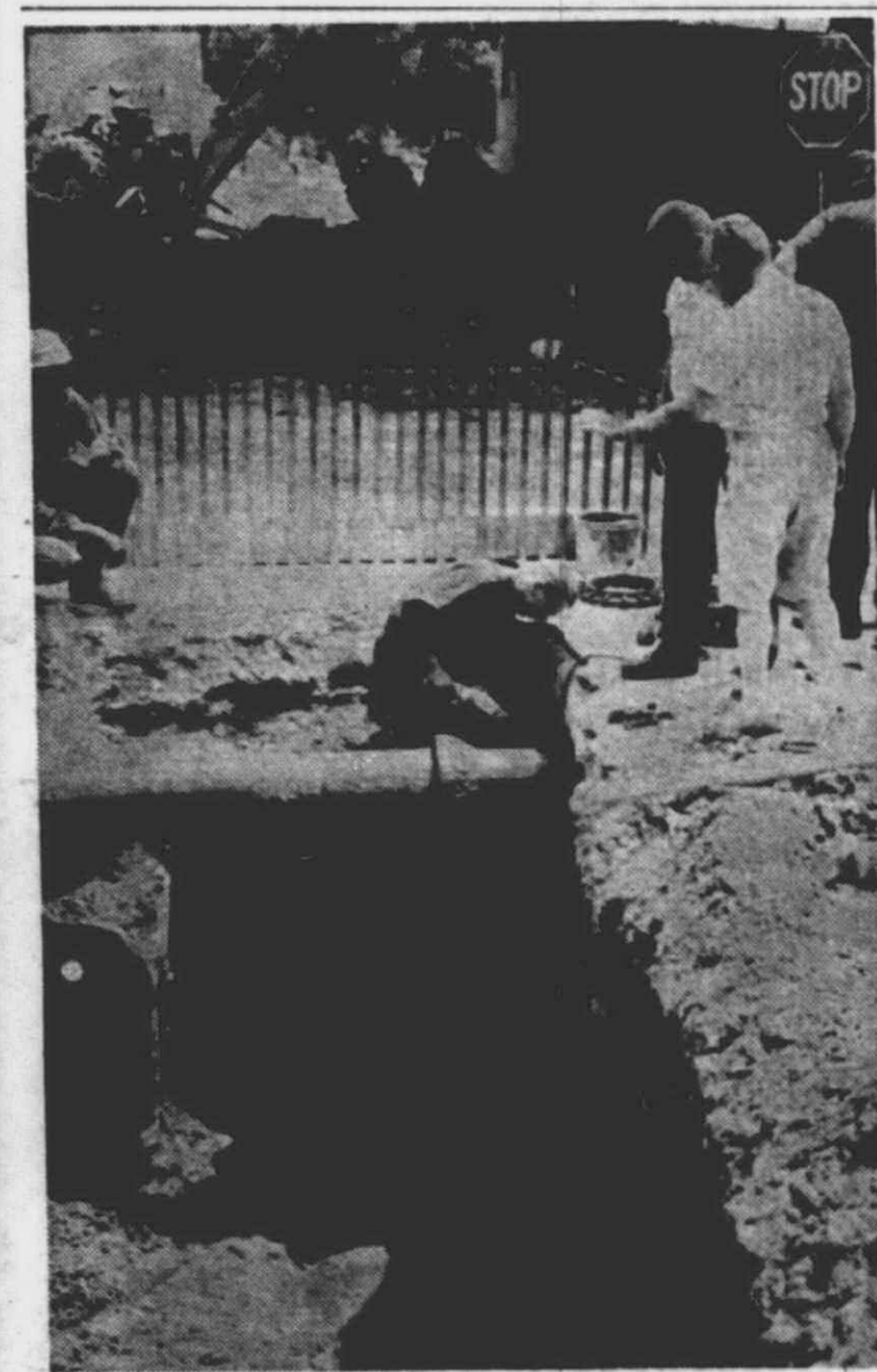
IT TOOK 37 MINUTES for a crew to install an eight-inch water main from the Plymouth system to the Haller Manufacturing Plant on Northville Road last Saturday. The plant was without water only a few minutes during the cutover, thanks to the co-operation of the Plymouth Township and City Fire Departments. DPW Supt. Joseph Bida is shown watching workers making the final connection — water flowed through the main within minutes.
