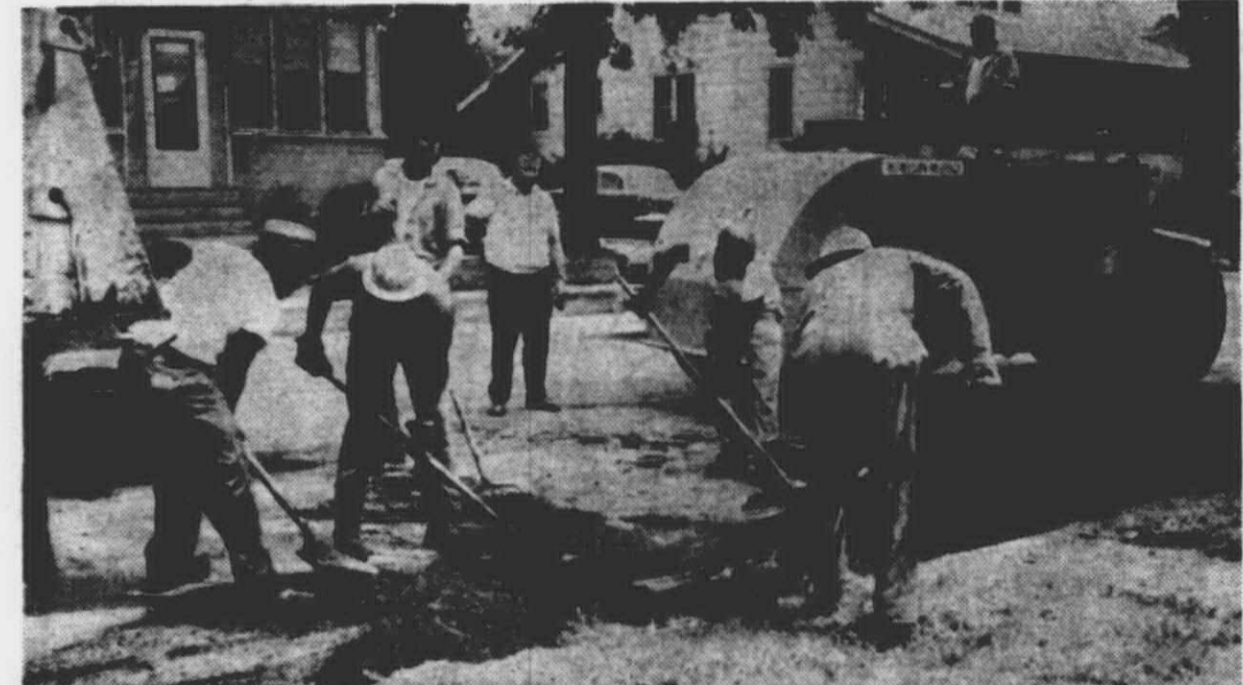
SATURDAY WAS ANOTHER workday for Plymouth's DPW Supt. Joseph Bida who was busy checking progress of work on the street improvement program. (Below) Bida watches workmen on the project at the corner of S. Harvey and Maple. (Above) He watches a crew placing a blacktop covering on Farmer Street between the C&O Railroad and Starkweather.
