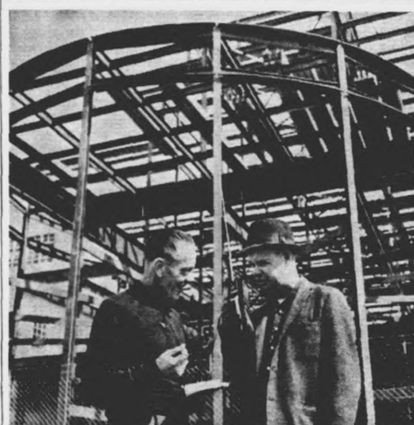
STUDYING STEEL CONSTRUCTION overhead are Bill Bettendorf, director of parking for the Detroit Race Course, and Building Supt. Dave Schaarsmith (right) as they look at the framework of the new $2.5 million clubhouse. Present plans call for the project to be completed by mid-July, well in advance of the August opening of the DRC's 84-day meeting.
