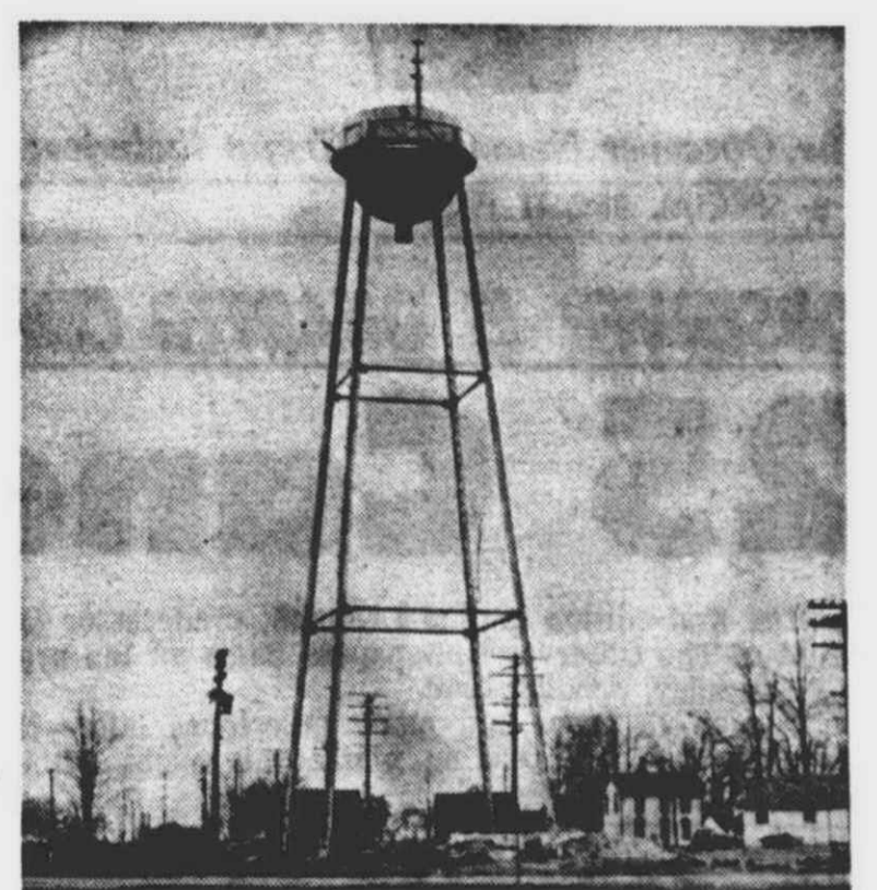
OLD WATER TOWER, which is shown in the process of being torn down in this photograph, once stood on the corner of Five Mile and Farmington Roads. This and the other photographs on this page were kindly lent to The Observer by Mrs. Elizabeth Donnelly, who has lived in the city for more than 30 years.
