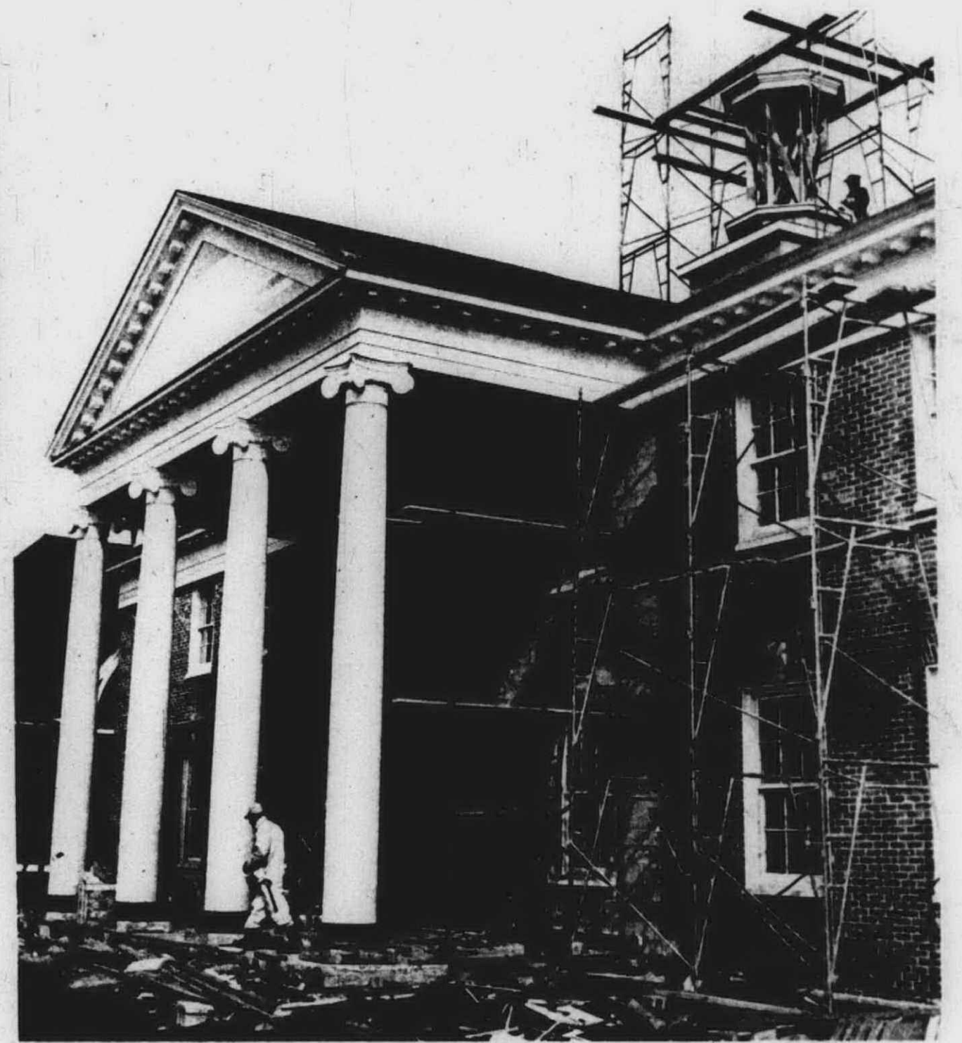
AS THINGS PROGRESSED on the new building, it took a semblance of its final shape. Here, painters' scaffolds are in place—next to the towering column which set the new building front off.
