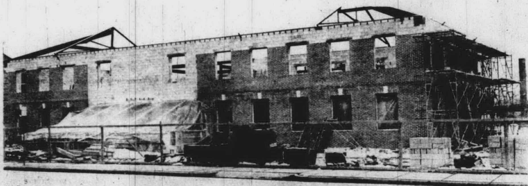
AS THE NEW building continued to grow, brick was put in place and the roof started to go on. General Contractor Ernie Burger kept his men working whenever they could during the winter to complete the project on schedule.
