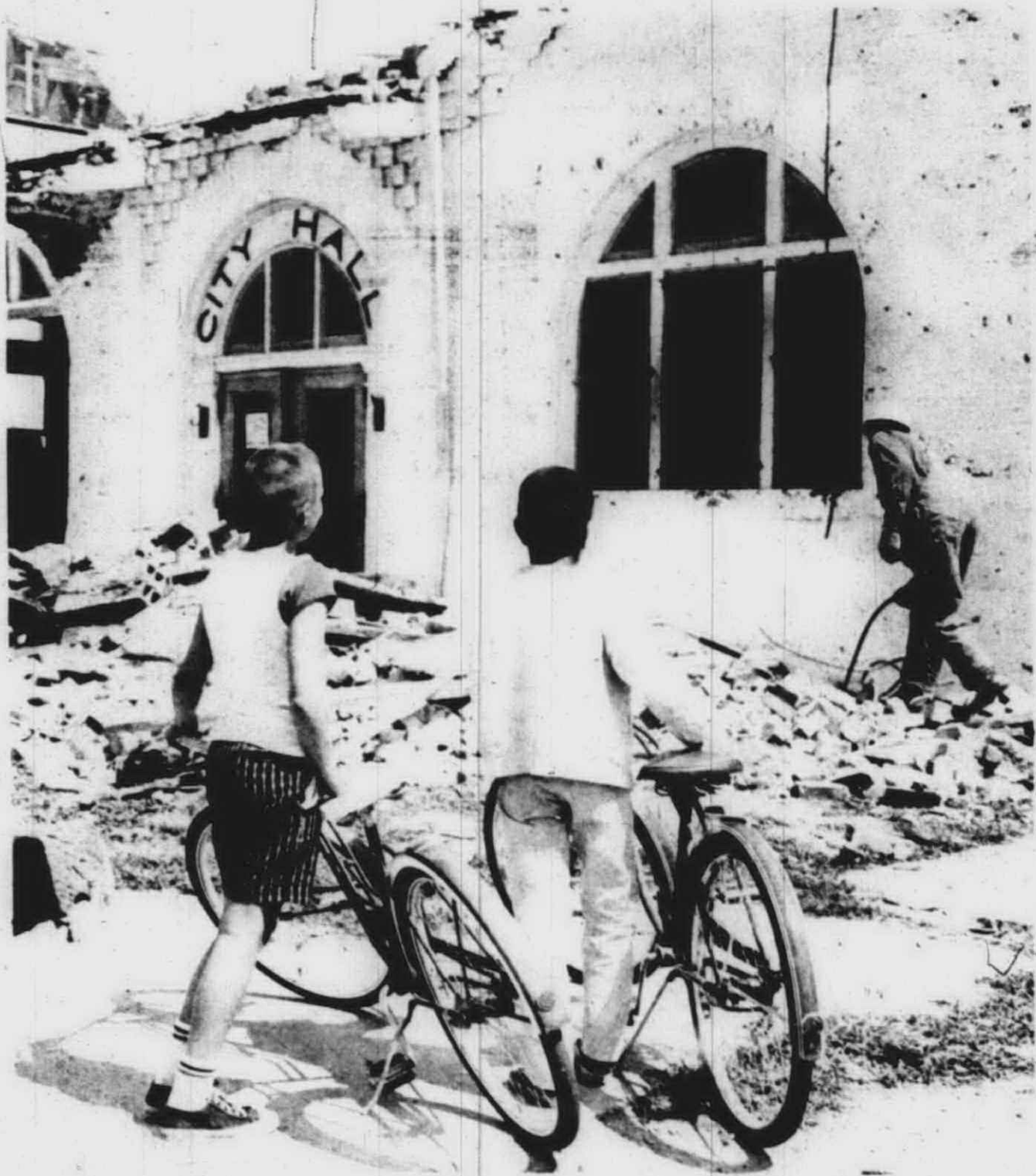
WATCHING with curiosity were these bike-riding Plymouth youngsters as the Old City Hall was torn down. Perhaps they were wondering if their children will live to see the new structure worn out and replaced.
