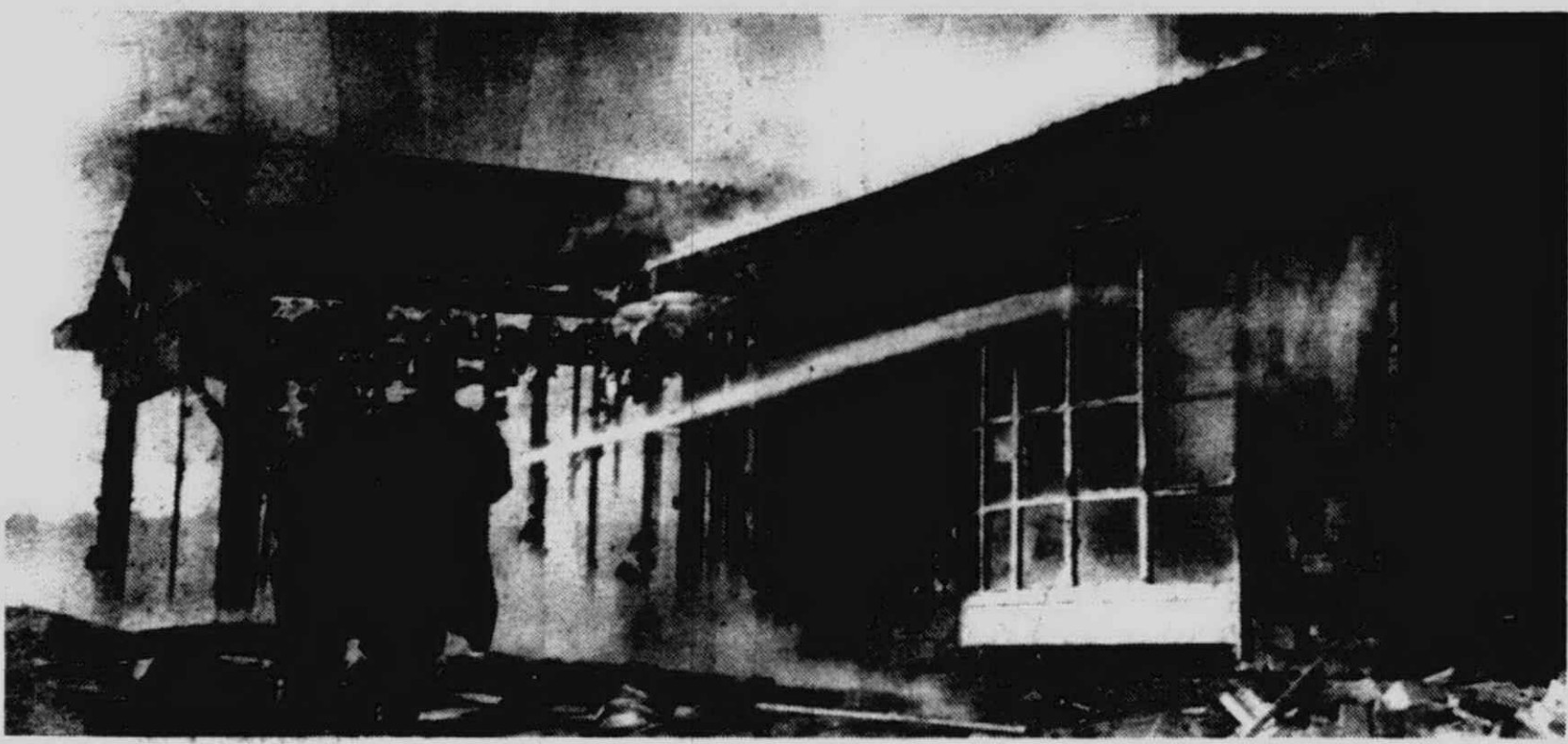
A PARTLY-COMPLETED new home in Lake Pointe Village went up in a flash of flames one day last summer and Township firemen had
