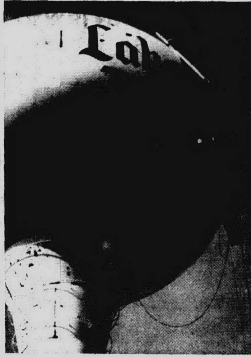
THE 400,000-gallon Lake Pointe water storage tank got a new coat of paint last week at a cost of $1,800. Here, workmen hover on scaffolding as they re-paint the lettering on the tank. The water tank is 135-feet high and measures 55-feet in diameter around the widest portion. It was last painted six years ago.
