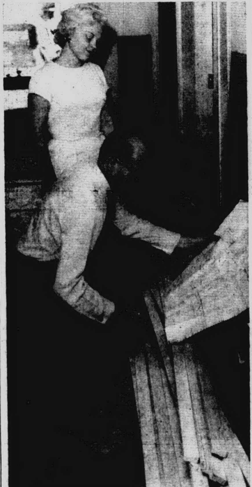
HUGH JARVIS GIFTS, on Ann Arbor Tr., is undergoing extensive remodeling this week. Changes include complete paneling of the walls and the incorporation of a beamed ceiling. Here, store owner Hugh Jarvis and assistant manager Evelyn Bailey study the plans for the project, which is expected to be completed next week.
