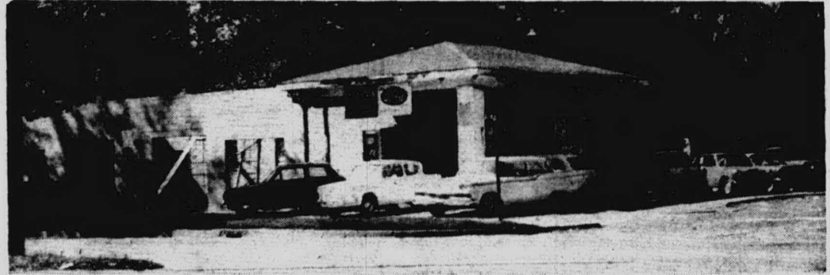
CONSTRUCTION of Joseph Stadnik's new English Ford showroom is underway at the corner of Main and Linden Sts. Utilizing an existing building that previously housed Flagg McCartney's service station, Stadnik is adding new showroom space in preparation for the official opening of his agency. Stadnik previously was in
