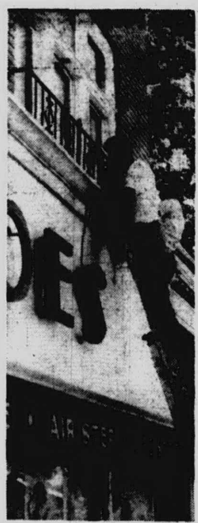
COLONIAL exterior of the Connor Building, at Main St. and Penniman Ave., is fast nearing completion. Here, workmen install wrought iron railings around second story windows of the building. Owner James Houk states the colonialization will be done sometime next month.
