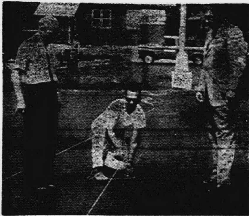
STRIPING of the central parking lot in the Plymouth Downtown Business District started last week under the supervision of city department heads. City Engineer Stan Besse (left) watched Manny Martin, of the Martin Striping Co., make a mark with a chalkline while Director of Public Service Ken Fisher (right) looks on.
