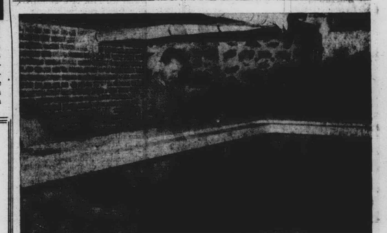
A RATHSKELLER-TYPE cocktail lounge will open in the basement of Fellows Creek Inn about Sept. 27. Workmen this week are putting the finishing touches to the remodeling project. The cocktail lounge will be named "Elliot's Ness-t." Here, a workman is sanding the terrazzo-tile bar top. Note the original field-stone foundation against the rear wall and the matching field-stone along the front of the bar itself.
