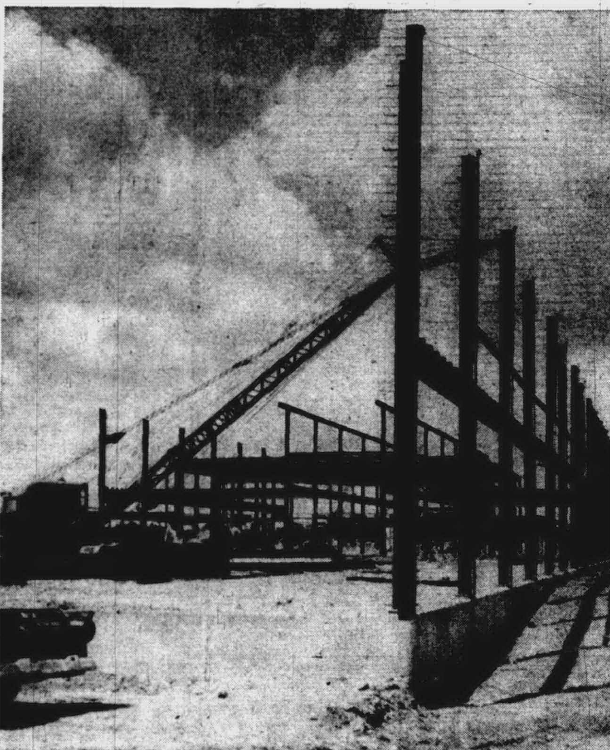
MAKING ITS appearance on the horizon is the new junior high school at Ann Arbor Trail and Sheldon Rd. Structural steel is this week being erected for the
