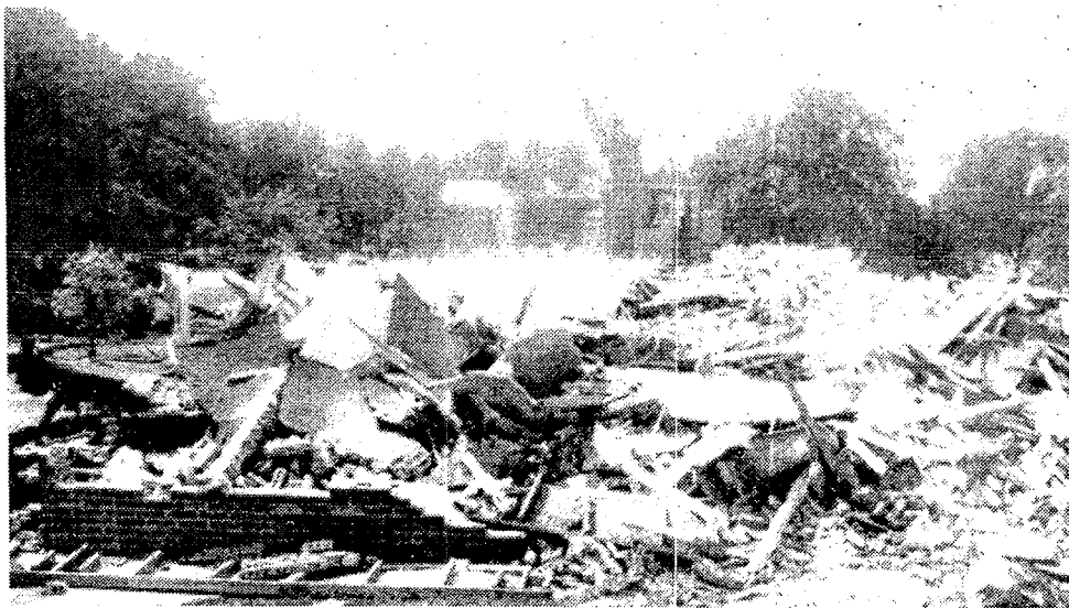
Make way for produce... Bulldozers began tearing down three buildings at Plymouth Square Apartments Monday to make room for a new Kroger store. The Kroger store currently located at Ann Arbor and Sheldon roads will be torn down as well when the new larger store is built. (Crier photo by Scott Goodwin)
