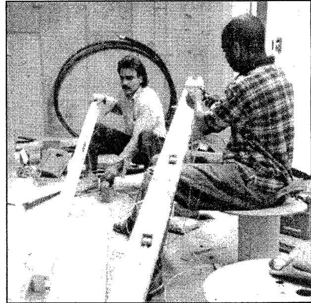
Before the lights can go on, they've got to go up: Nick and Romelo from Duran Electric (at left) wire two of the hundreds of fluorescent light fixtures being hung in the library's lower level. Nearby, Sam Lalonde and Marvin Jackson (below) tangle with a few coiled feet of the more than 12 miles of communication lines that will connect the library's computers and internal networks.
