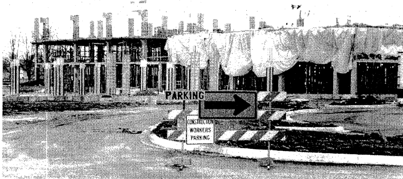
Yazaki North American's $60-million, 400,000 square-foot headquarters is one of a number of major industrial and commercial investments companies have made in Canton this year. (Crier photo by R. Alwood, Jr.)
