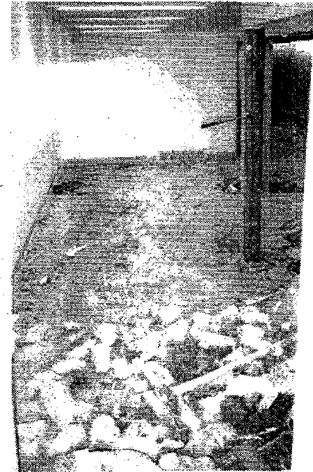
Four months of strenuous work went into remodeling the lower level of Gabrial's, which had hosted many businesses over the years, including a stable in 1893 to, most recently, Little Hang Ups. A picture from the early stages of reconstruction shows some of the 26 yards of field stone removed by conveyor belt, as well as a workman's hammer (Crier photo courtesy of Larry Bird).
