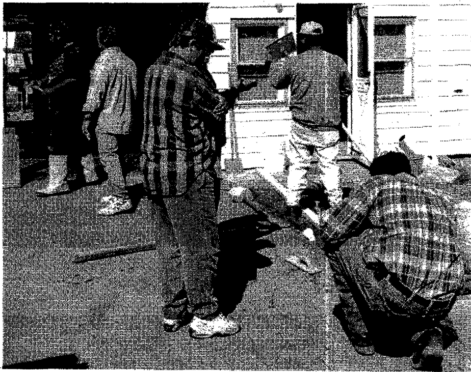
Dozens of Rotary members and volunteers came together to renovate this Plymouth Township home. (Crier photo by R. Alwood Jr.)
