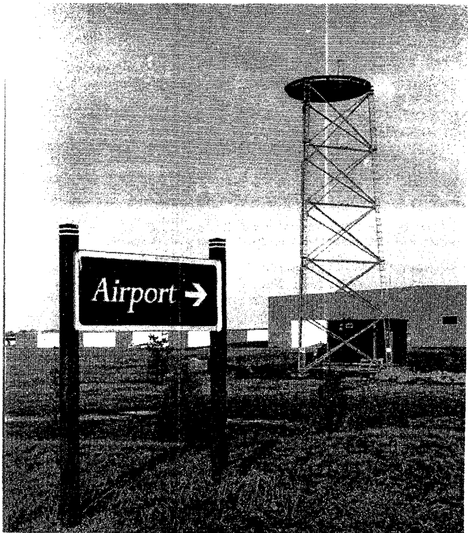
Construction on Channel 7's Doppler radar tower at Mettetal airport is nearing completion. (Crier photo, R. Alwood, Jr.)
