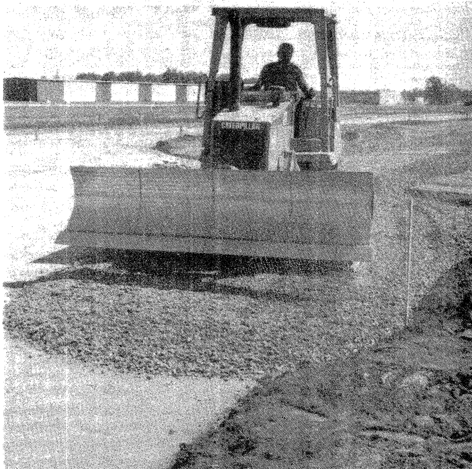
While the Canton-Plymouth Mettetal Airport Advisory Board is chosen, work crews continue to construct the new runway at the airport. (Crier photo by Rob Kirkbride)
