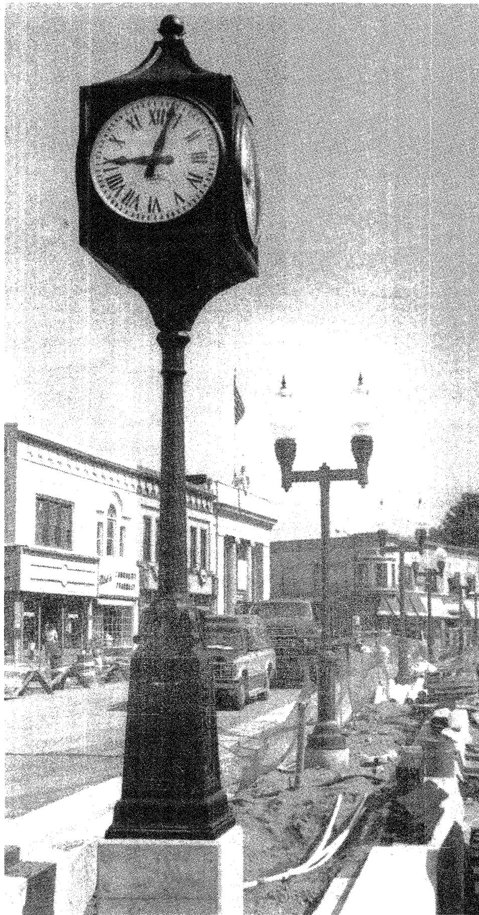
The Guenther Clock, now located at its new home on the corner of Ann Arbor Road and Main Street, is expected to be turned back on soon. Electric crews are busy hooking up the power that will run the clock and the new streetlights. Forest Avenue construction is nearly complete with the final touches being applied this week. Construction continues on the Plymouth Streetscape project, with sidewalks along Main Street torn up this week. Construction on Main Street is expected to be complete by Fall Festival and should not disrupt the annual event. (Crier photo by R. Alwood Jr.)
